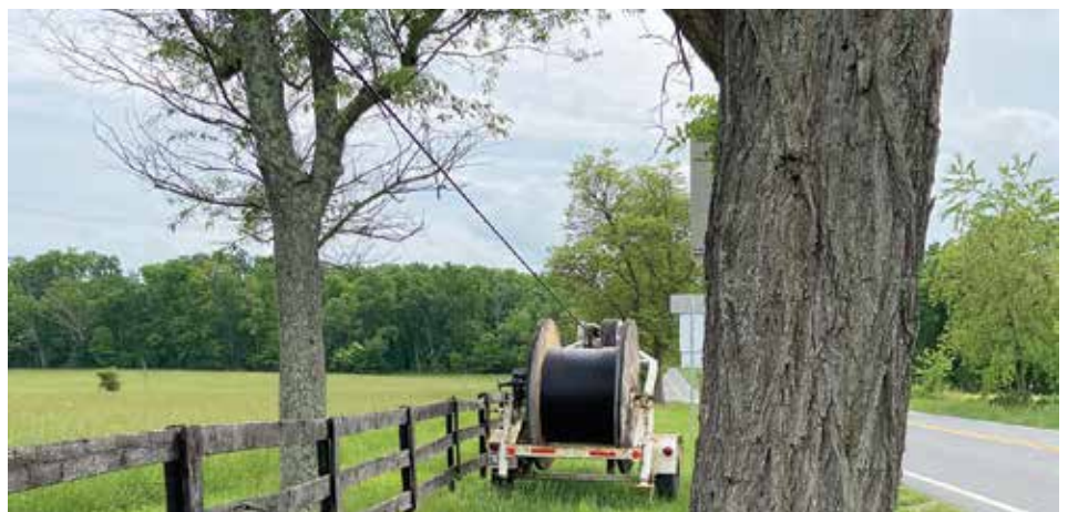
Fiber optic cable installation at the intersection of St. Louis and Foxcroft roads near Unison.
